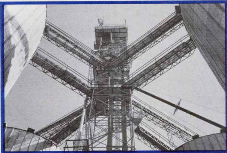
AG REMP SERVICE, 1750 BROADWAY WATERLOO, IA 50703 OVER 1,500 FT OF 7,000 BU/HR IGUANA CONVEYOR
